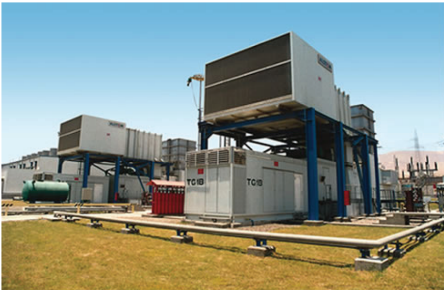
Fig. 3. General view of a gas turbine power plant.
